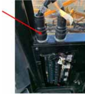
FIGURE 5. X-59 Bulkhead Connector (Located Near Front of Cab)
